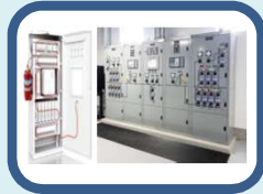
ELECTRICAL ROOM-SAFETY SOLUTIONS
