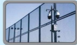
Fence with CCTV and Alarm Integration
