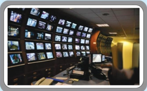
CCTV Control Room
