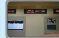
Power Generation Display
