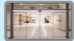
Automatic Sliding Door (Club House)
